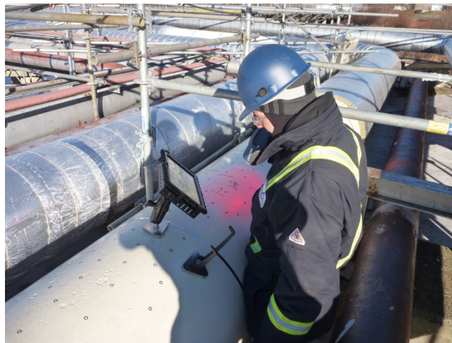
Figure 2 : Pipeline inspection with Handyscan3D laser scanner and real-time visualisation on a tablet
